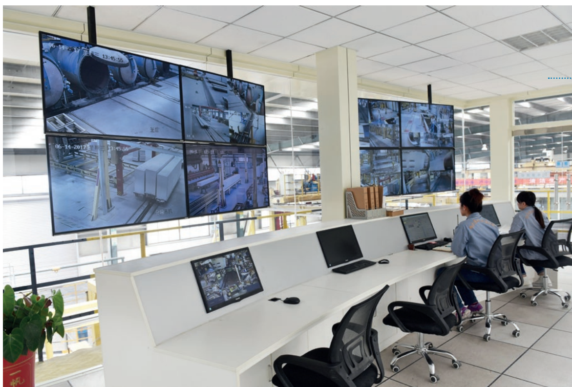
Central integrated control room.
